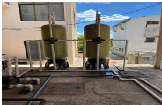
Fig. No. 2 STP plant
