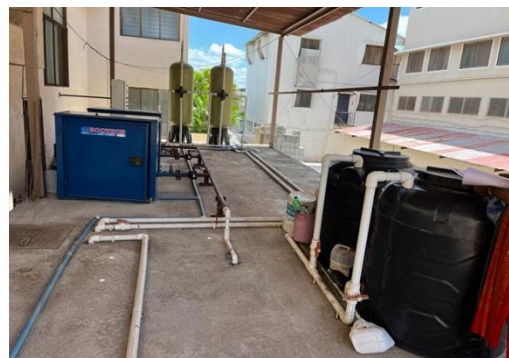
Fig. No. 3 STP plant
