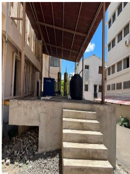
Fig. No. 1 STP plant
